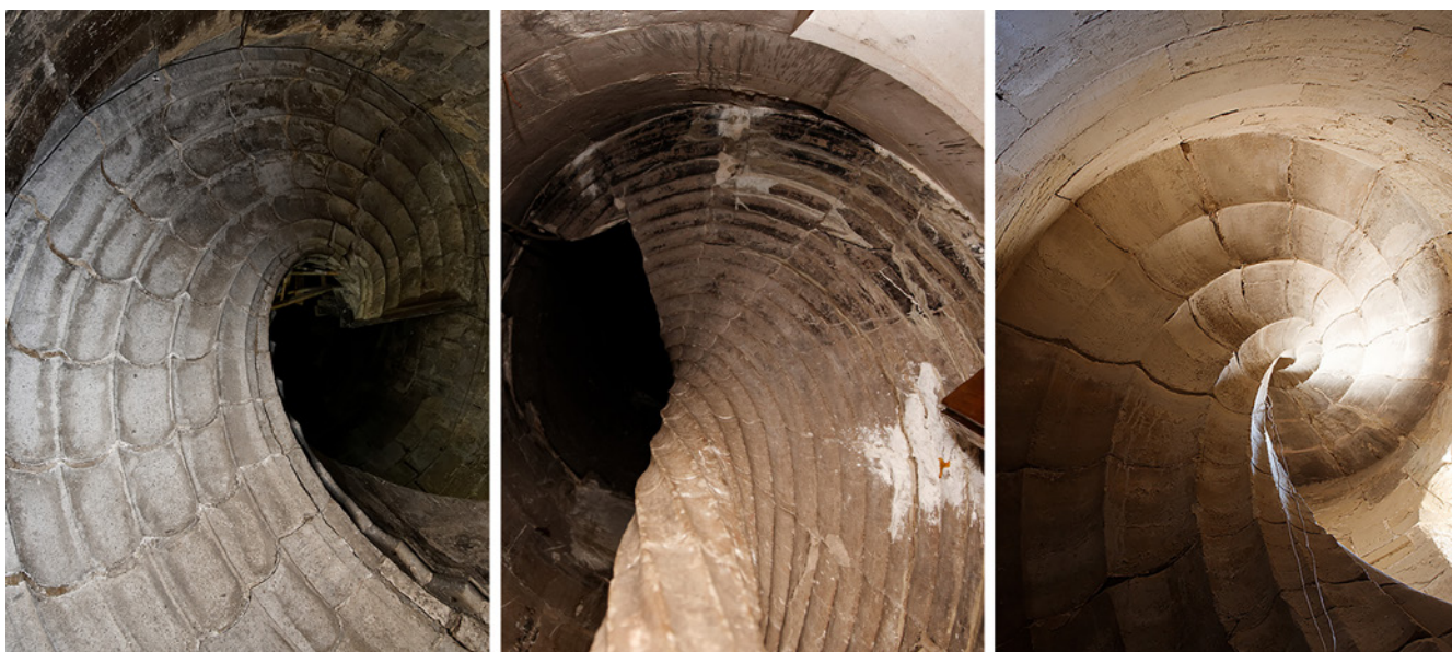
Figure 6. Left. Intrados surface of the staircase of Honor. Center. Intrados surface and flute newel of the staircase in the Sala de Baroni. Castenuovo, Naples. Guillem Sagrera. Right. Intrados surface of the staircase in the Cathedral of Cuenca, Located in the ambulatory with the aim of giving access to the roofs of the Cathedral (Images by the authors).
