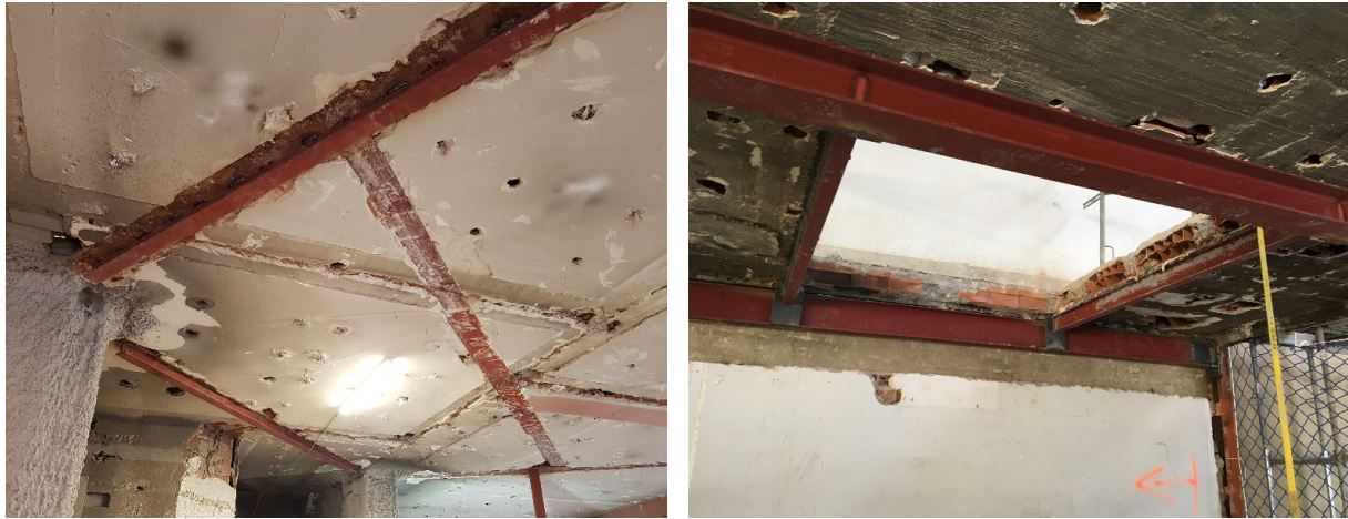
Fig. 6: a) Steel beam reinforcement intervention. b) Intervention of new opening with new structural elements
