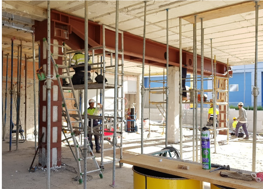
Fig. 5: Shoring and reinforcement intervention in columns
