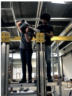
Fig. 255 Hormigonado experimental de una columna, A Prototype Pavilion in Textile Reinforced Concrete , 2019, Suiza.
