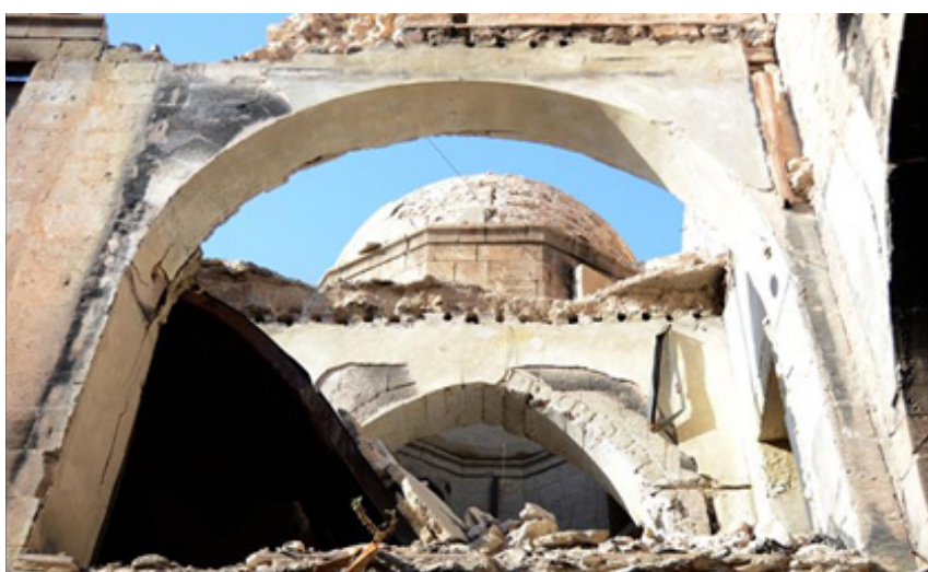
Severe damage on St. Markourkas Church (Anadolu Agency, 10/03/2015)
