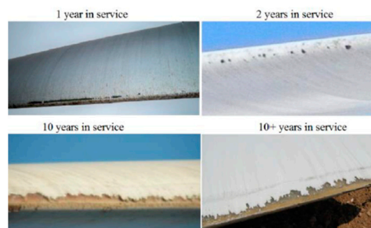
Figure 1. Examples of leading edge erosion across a range of years in service, from [1].
