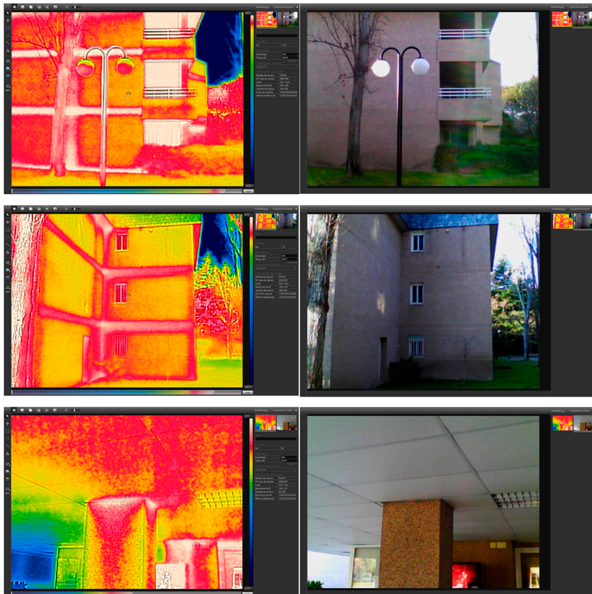
FIGURE 4 Thermographic images of different areas of the existing building.
